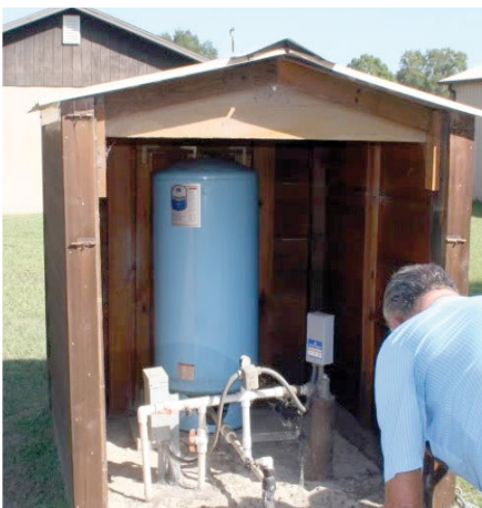
Home well water system
