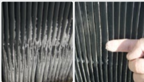
Cooling tower grids
