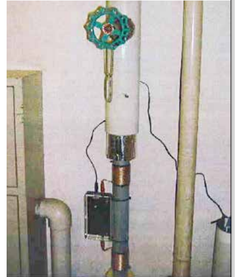
Vulcan 5000 was installed in the factory kitchen
