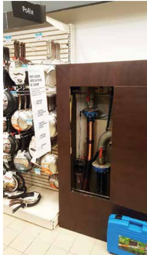
Vulcan S25 was installed in the water main to treat the whole building.
