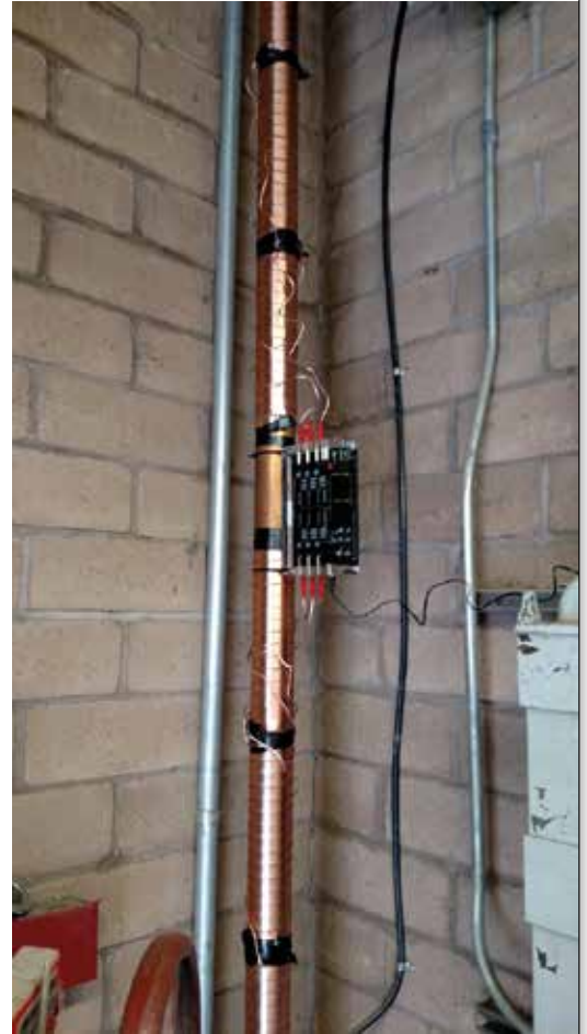
Vulcan S100 installed on the main water line
