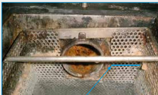
Usual level of standing water.
