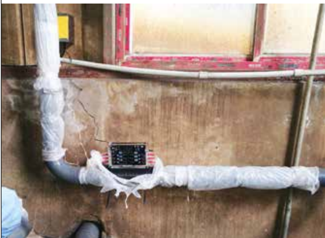
Vulcan S100 was installed in the sewage room to treat the sludge dewatering machine.
