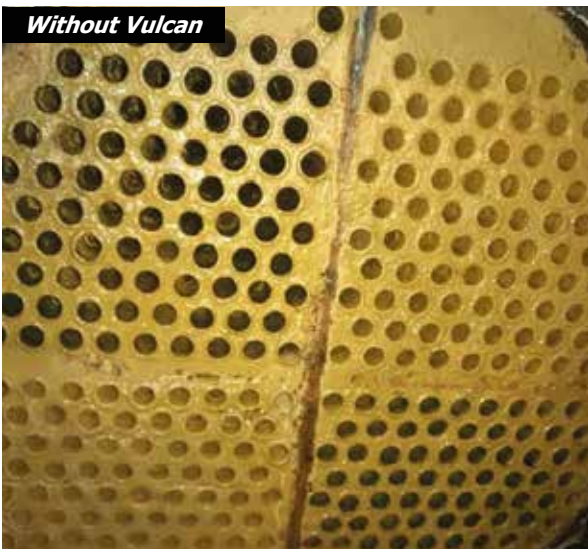
Before installing Vulcan, the scale was very thick and hard in the heat exchanger tubes.
