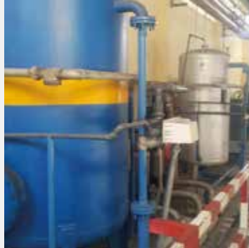
Stopped water softener
